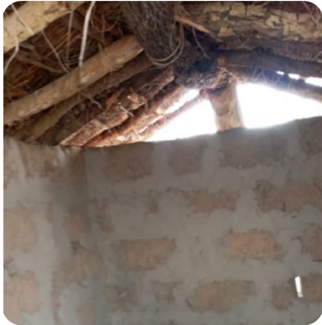
Gap between the roof and walls
