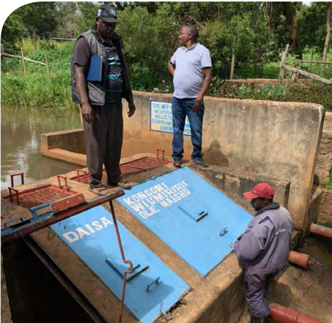
A self-regulating water intake constructed and managed by the Ngusishi WRUA.
